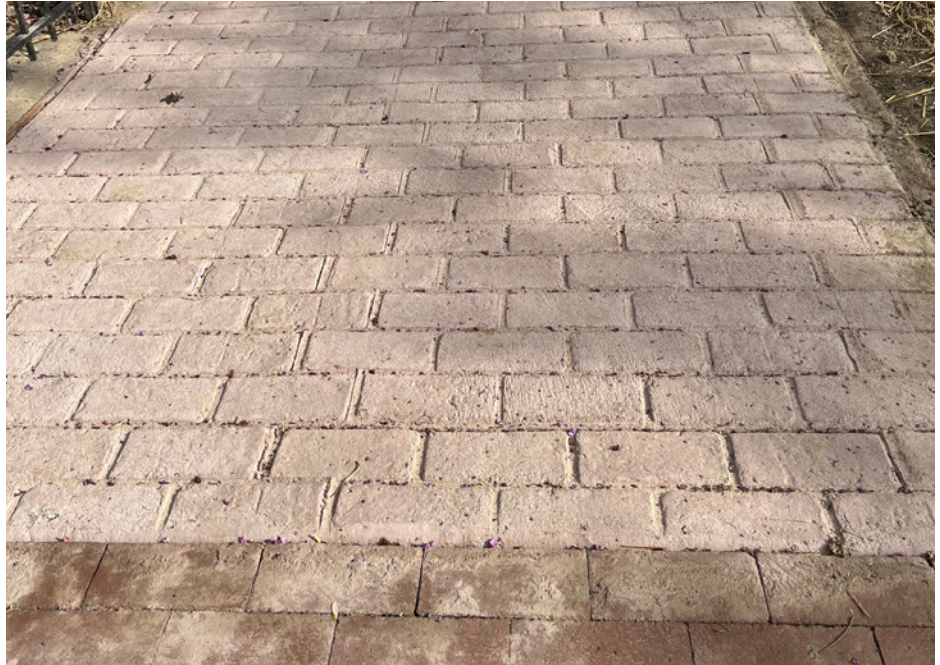
The stamped concrete section is at the top of this photo, contrasted with existing brick at the bottom. The trial is in the 700-800 blocks of 10 St. NE. If you have the chance to check it out, Council Member Allen would like your feedback at Charles@charlesallenward6.com .
